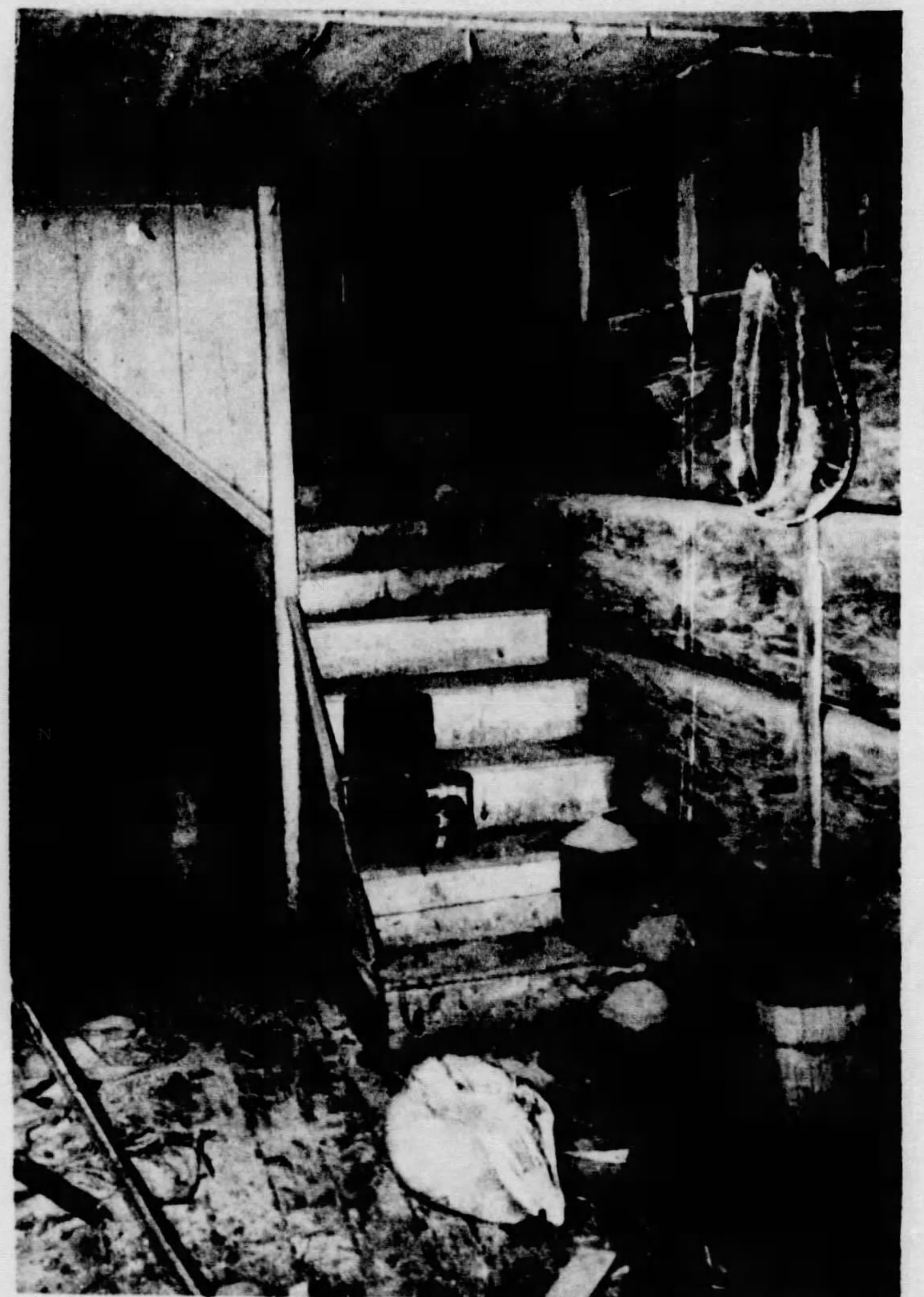
Inside the house the log walls once were sheathed in wide pine boards covered with "speckled" paint.
