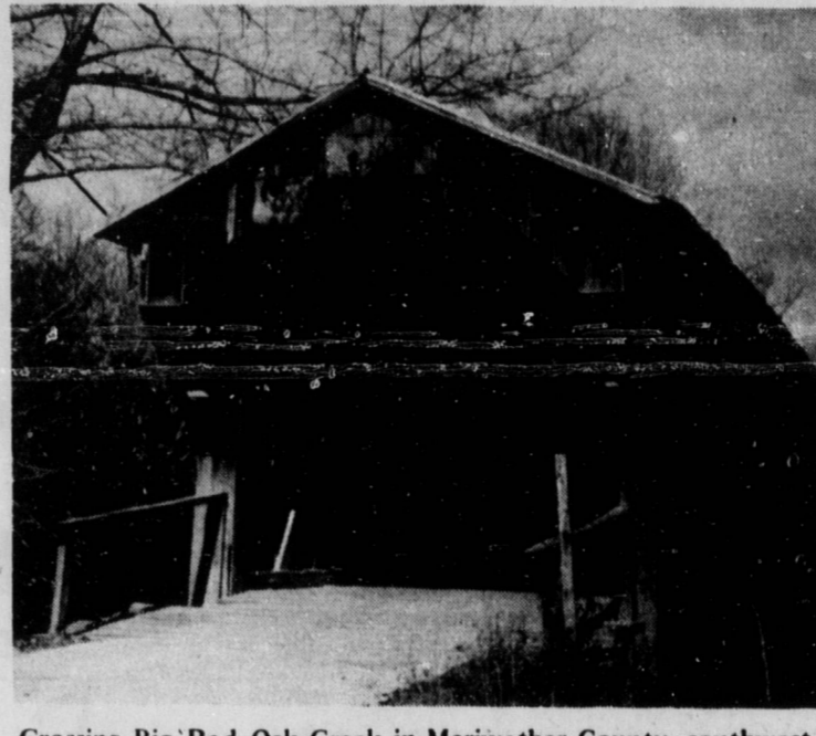
Crossing Big Red Oak Creek in Meriwether County, southwest of Atlanta, is a partly-covered 412-foot bridge, longest of Georgia's antique bridges. (PRN)
